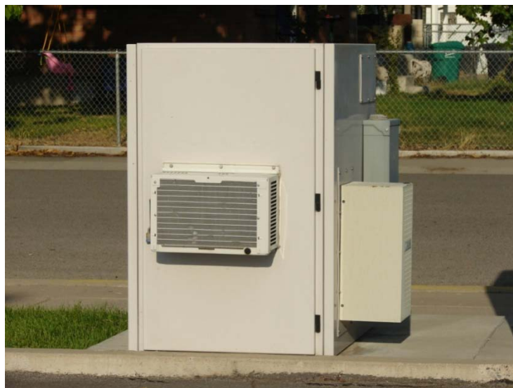
Figure 10 – iProvo Demonstration Area Cabinet
