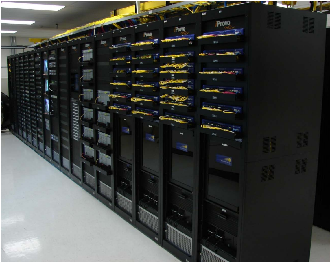
Figure 28 - Provo Network Core and Headend
